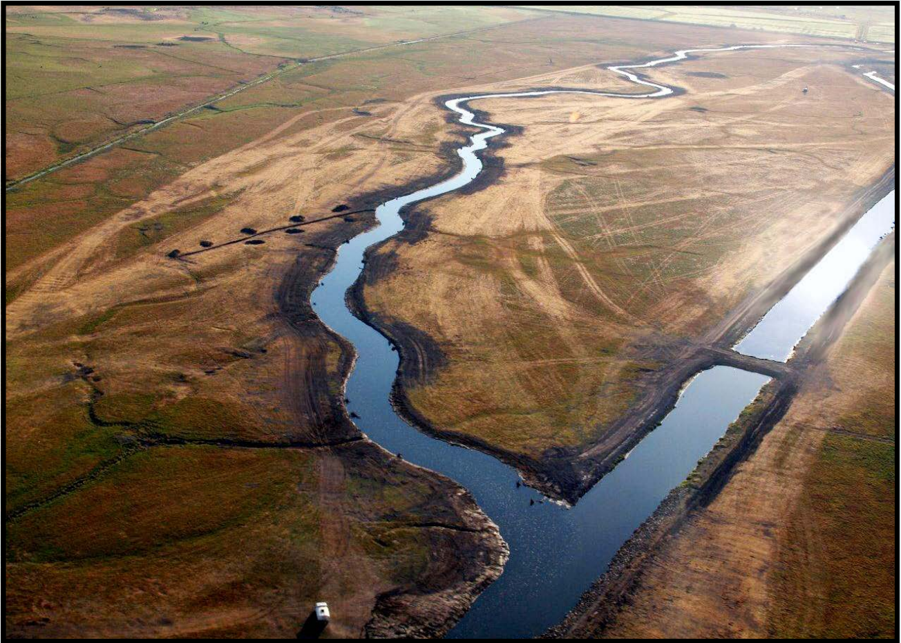
View of South Fork Sprague River Channel Realignment; the newly completed South Fork Sprague River is on the left and the former flow path of the South Fork Sprague River is on the right.
