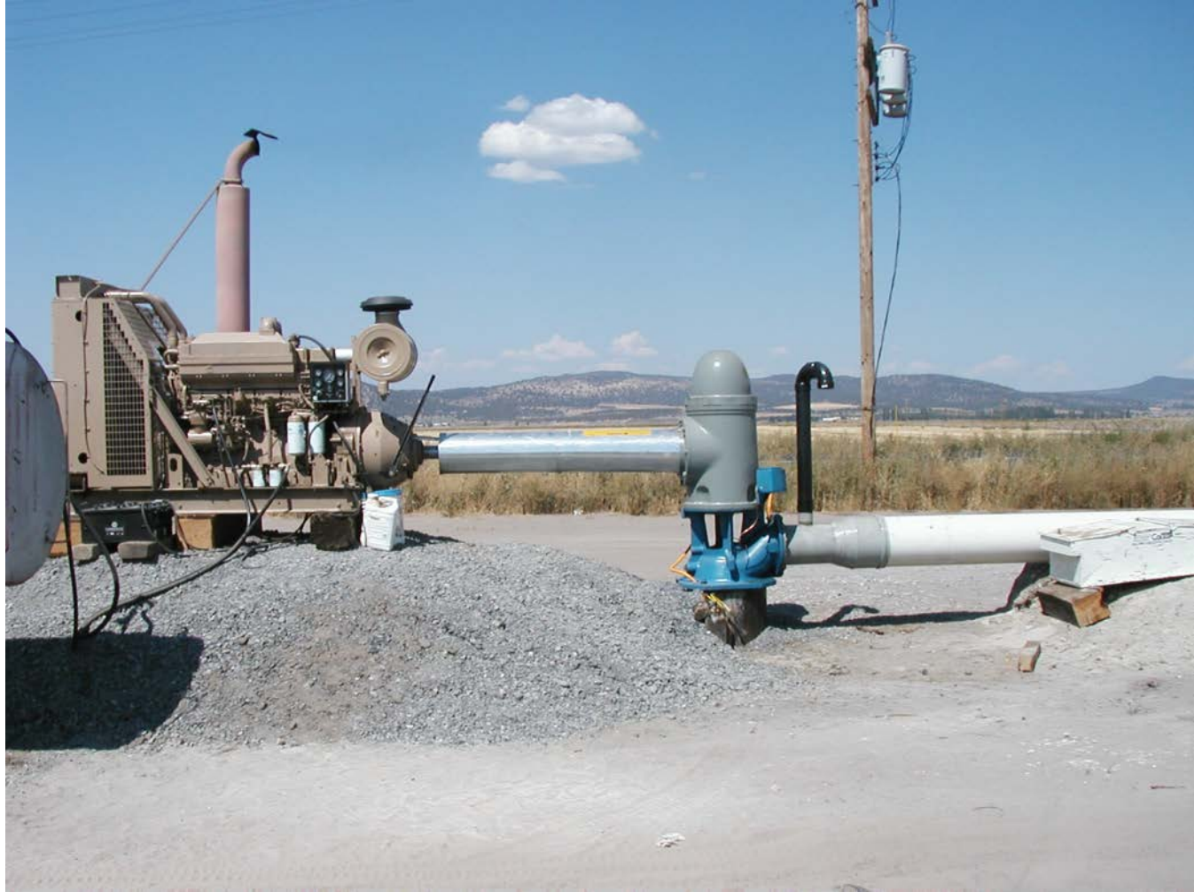
Figure 3-12. One of many irrigation wells installed in 2001 to supplement surface-water supplies depleted by drought. (Photograph by Charles Palmer, USGS.)
