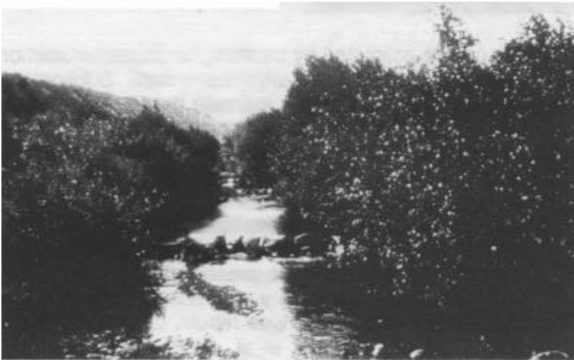
Top: Stream before treatment. Middle: After installation of boulder weirs, at higher flow. Bottom: Streamside replanting beginning to mature.
