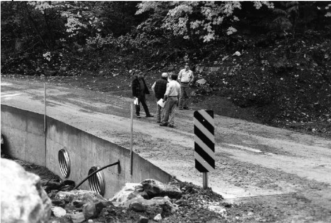
Figure A5-26. New cement ford on Kelsey Creek installed by Klamath National Forest with flood relief money. This approach should reduce long term maintenance and prevent sediment input into Kelsey Creek. October 1997.
