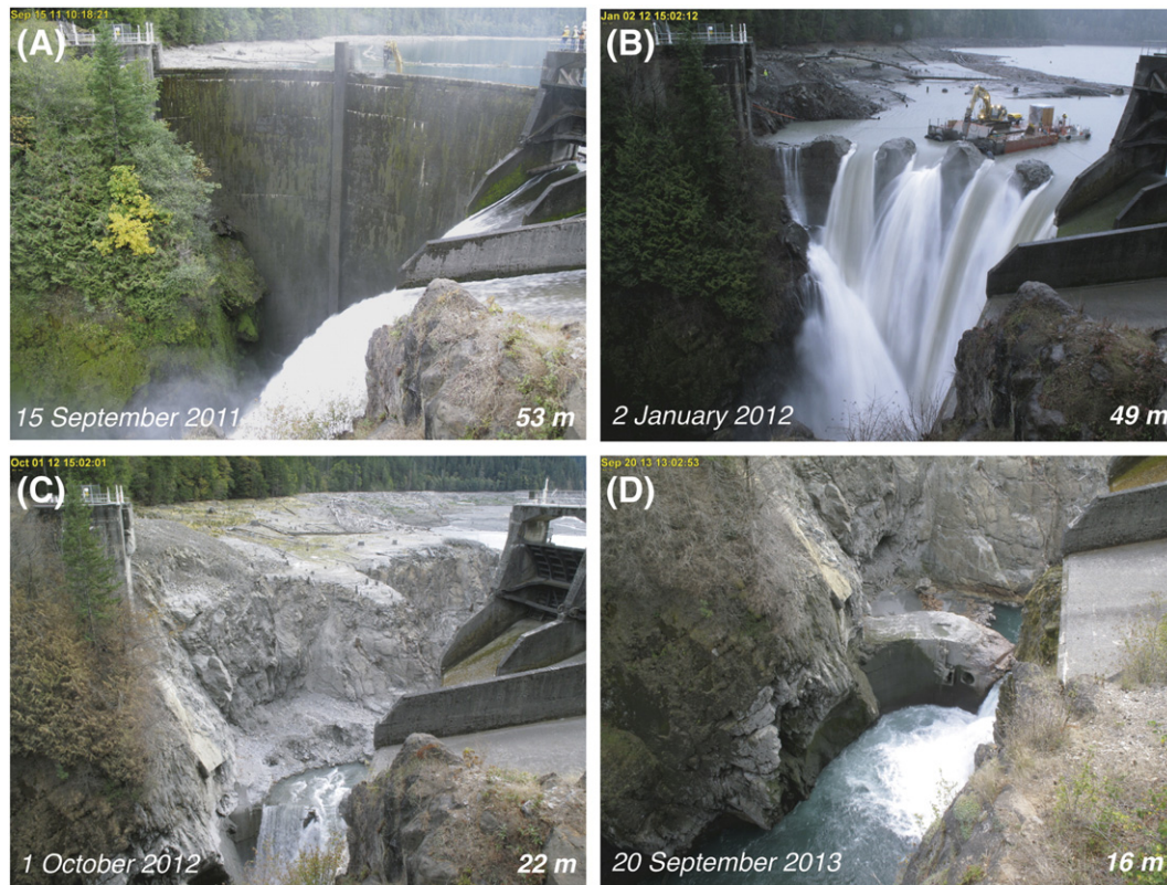
Fig. 3. Decommissioning of Glines Canyon Dam as shown by photos from National Park Service time-lapse cameras. Dates and heights of the water surface above the original channel bed are shown in each photo. (A) The initiation of dam removal in mid-September 2011. An excavator floating on a barge and equipped with a hydraulic hammer can be seen near the center of the dam. (B) After 3.5 months the upper portion of the dam had been removed, and river discharge no longer could be passed through the spillways in the foreground. (C) After 1 year the reservoir sediment delta had prograded to within 100 m of the dam. (D) Although the reservoir delta prograded to the dam during high flows of October 2012 and sediment could spill directly into the channel below, the river had low turbidity during the summer low flow season of 2013. Photos provided by Erdman Video Systems in collaboration with the National Park Service.
