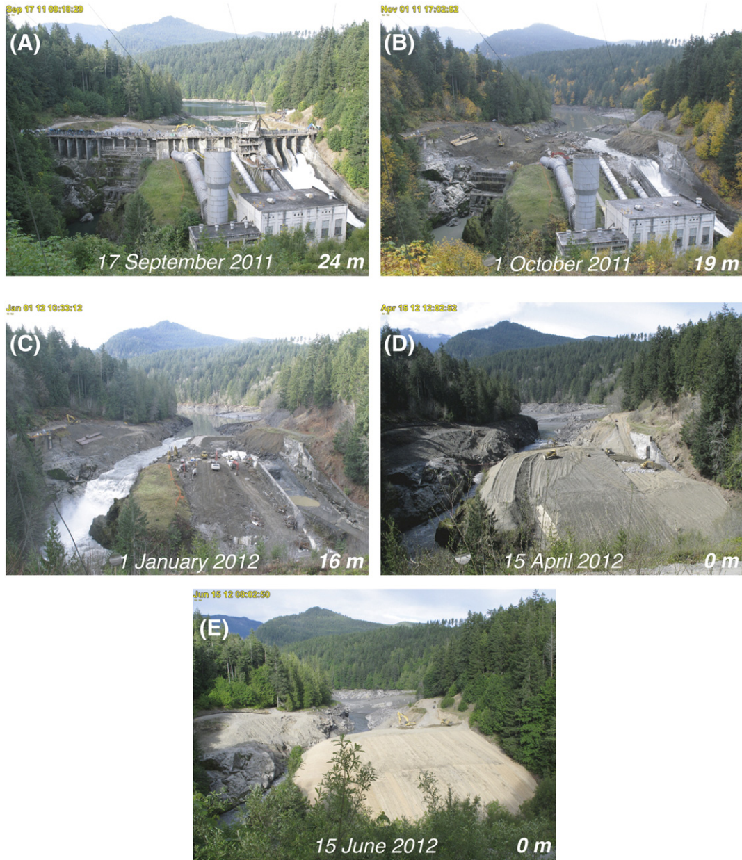
Fig. 2. Decommissioning of Elwha Dam as shown by photos from National Park Service time-lapse cameras. Dates and remaining heights of the water surface above the original channel bed are shown in each photo. (A) The initiation of dam removal in mid-September 2011. Removal of the dam involved successive excavation of the spillway (B; right side of photo) and the dam structure (C; left side of photo) and multiple managed shifts using earthen cofferdams to alter the river course through these waterways. (D) The Elwha River in the spring of 2012 following the final managed river shift into the excavated canyon. (E) Final graded hillside of the Elwha Dam site following dam removal. Photos provided by Erdman Video Systems in collaboration with the National Park Service.
