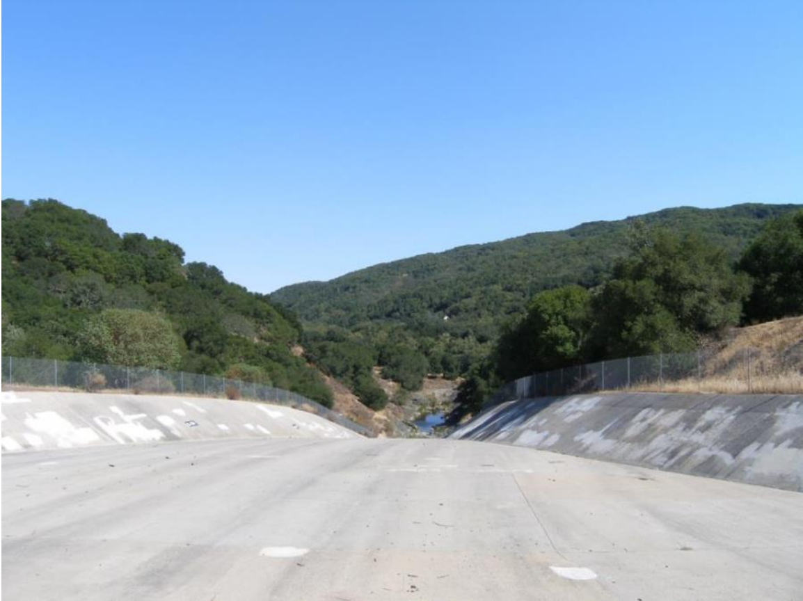
Figure 5. Uvas Dam on the Uvas Creek a tributary to the Pajaro River. Uvas dam blocks passage to historical habitats and should be evaluated for potential to provide passage and incorporate Pacific Lamprey into streamflow management decision-making. The photo is looking downstream from the top of the reservoir overflow channel. Photo taken in August 2013.
