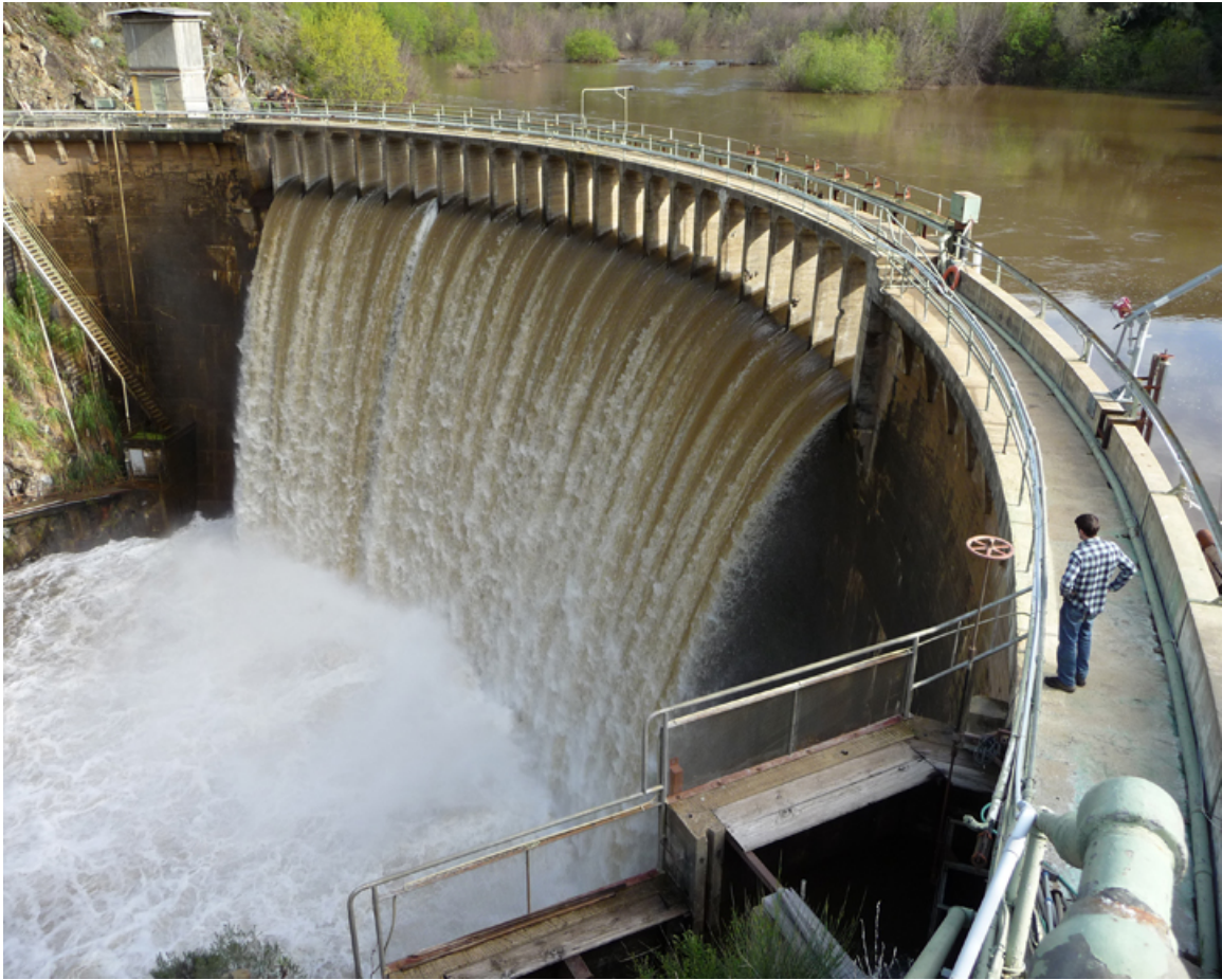
Figure 8. San Clemente Dam on the Carmel River. Passage above the dam will provide an additional 7 miles of mainstem habitat, an implementation action that is currently underway (Photo courtesy of the San Clemente Dam removal project).
