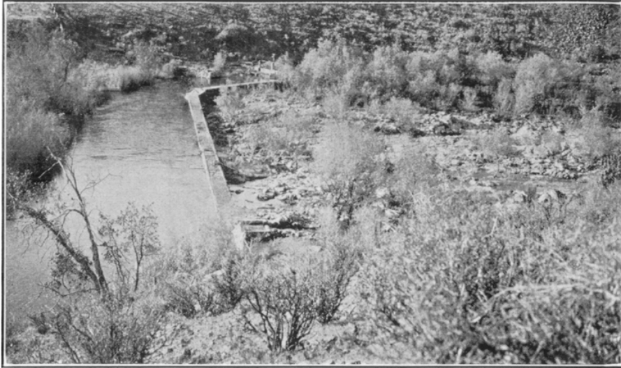
FIG. 18. Shasta River dam with fishway in the foreground and rocky streambed below. View taken from point 2 on map, figure 17.
