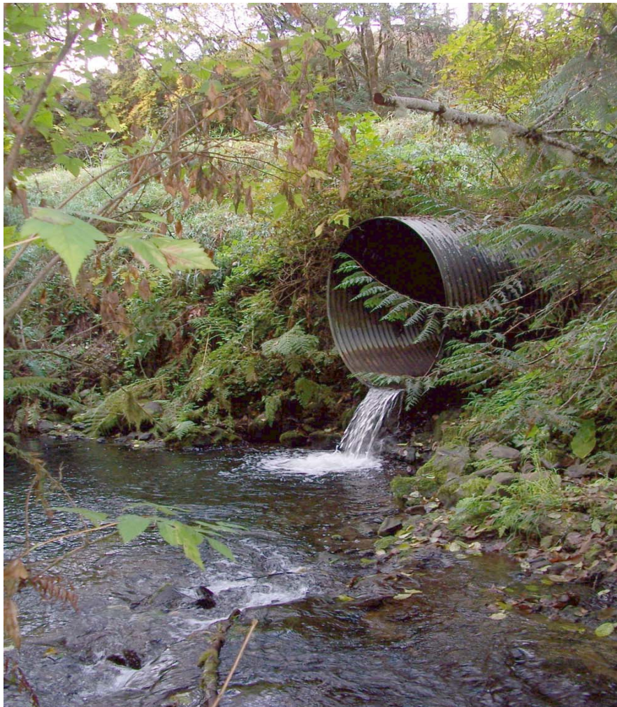
Fern Flat culvert at confluence of E Fork Dairy Creek & Campbell Creek
