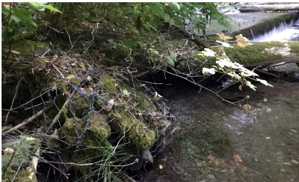
Figure 2-3. Previous restoration work completed on Cedar Creek, Lower Trinity RD. Gabion basket (cyclone-fencing baskets filled with rocks) in forefront with rebar-pinned full spanning large wood structures in background. Photo courtesy of Ely Boone.
