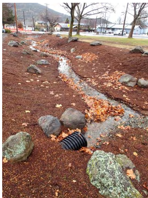
Figure 5.18. Evergreen Bioswale Project in 2015 before and during construction, and in 2016 after construction.
