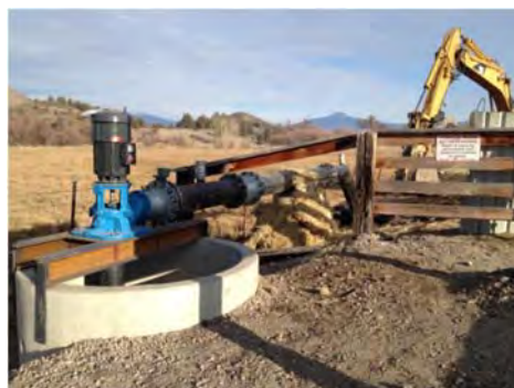
Figure 5.3. Pump and pipeline projects are designed to manage and reduce tailwater.
