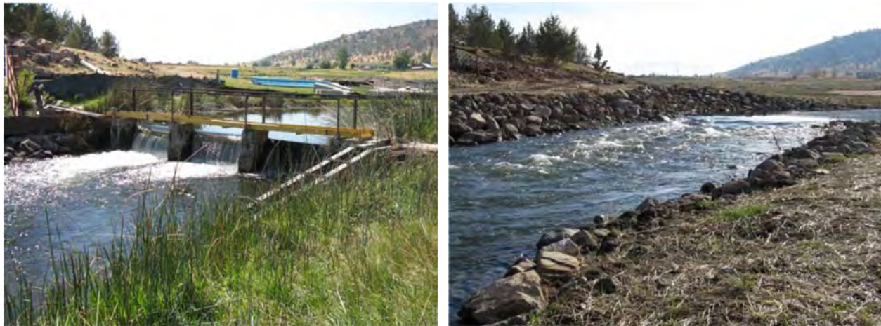
Figure 5.1. Shasta River Water Association Flashboard Dam fish passage improvement project implemented in 2008, shown in pre-project and post-construction photos.
