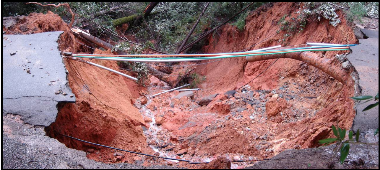
Figure 25. Road failure caused by diversion from plugged culvert on Mud Creek, Somes Bar, CA, during the 2006 flood event.
