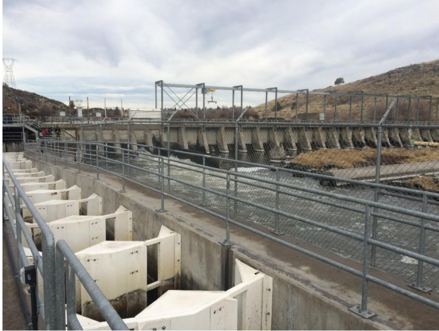
Figure 3-13. Link River Dam located at rkm 414.4 (rm 257.5) constructed in 1927 at the outlet of Upper Klamath Lake (background), and the associated fish ladder (foreground) constructed in 2005, specifically for the use by suckers, salmonids, and lampreys.
