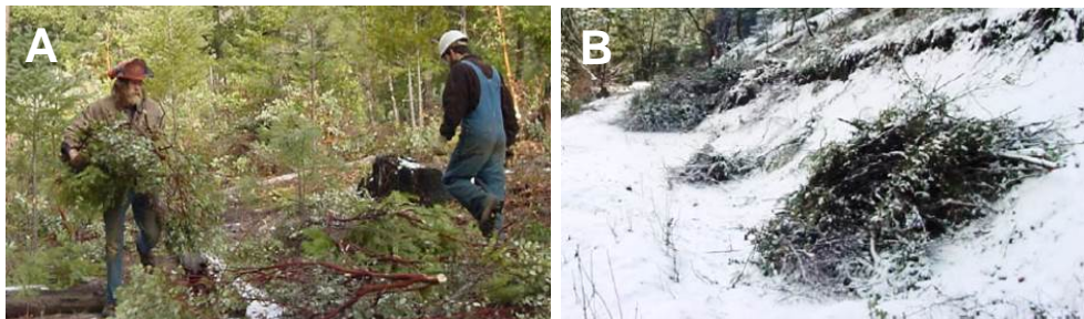
Figure 6-39: Workers carrying out manual removal (A) and stacking for disposal by controlled burning (B) of understory vegetation that contributes to increased fire risk in coastal forests. (USFWS / Villeponteaux and Greenberg 2005).
