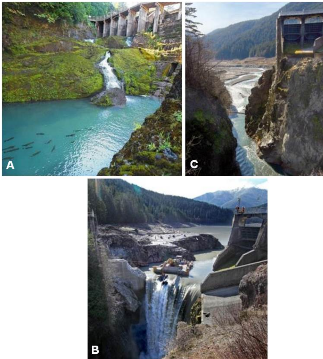
Figure 1-3: Photos of the Elwha and Glines Canyon Dam removal on the Elwha River. The photo 11 in (A) was taken in 2010 and shows adult Chinook salmon blocked in their journey upriver by Elwha Dam with no fish passage. Even after 100 years they persisted, circling at the face of the dam every spawning season, trying to get upstream. The 2012 photo 12 in (B) shows the partially deconstructed Glines Canyon Dam and Lake Mills. The dam is now removed and the Elwha River is free-flowing (C). A newly opened viewpoint perches on part of the dam's former spillway.
