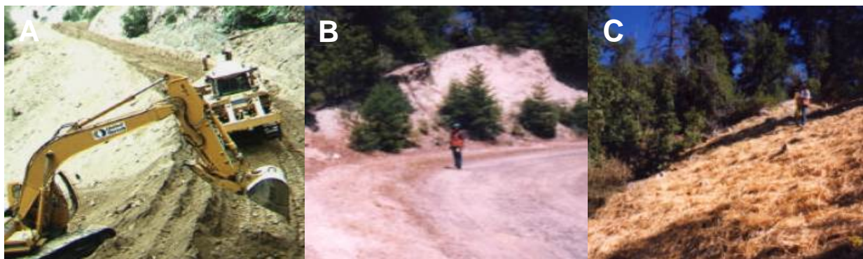
Figure 6-38: Road decommissioning along Steinacher Road in the Salmon River sub-basin. Fill excavated at some road segments (A) is used to backfill other through-cut road segments without fill (B), and is then covered with straw or mulch (C) to reduce erosion until vegetation can establish. Reproduced from NewWave 2001.
