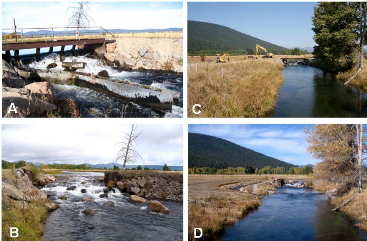
Figure 6-15: Photos of Sevenmile creek showing the main channel diversion before construction (A) and following its replacement with a rock weir during the project (B), as well as showing the entire main channel before construction (C) and following replacement of diversion structure, channel roughening, and the addition of a fish bypass on the left following construction (D). Photos reproduced with permission from Trout Unlimited.
